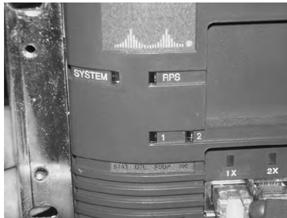
Figure 11.1 Front Panel Lights on a Cisco Switch
